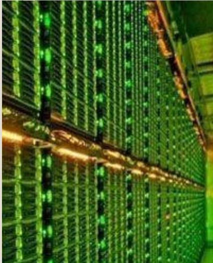
Green Data Center
